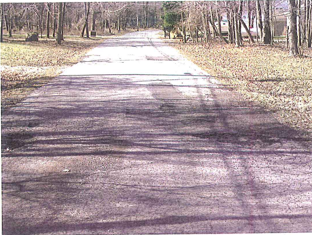
Picture 11 – Pavement Segment 321 (3366 Memorial Shoreway) CONDITION RATING NUMBER 3
