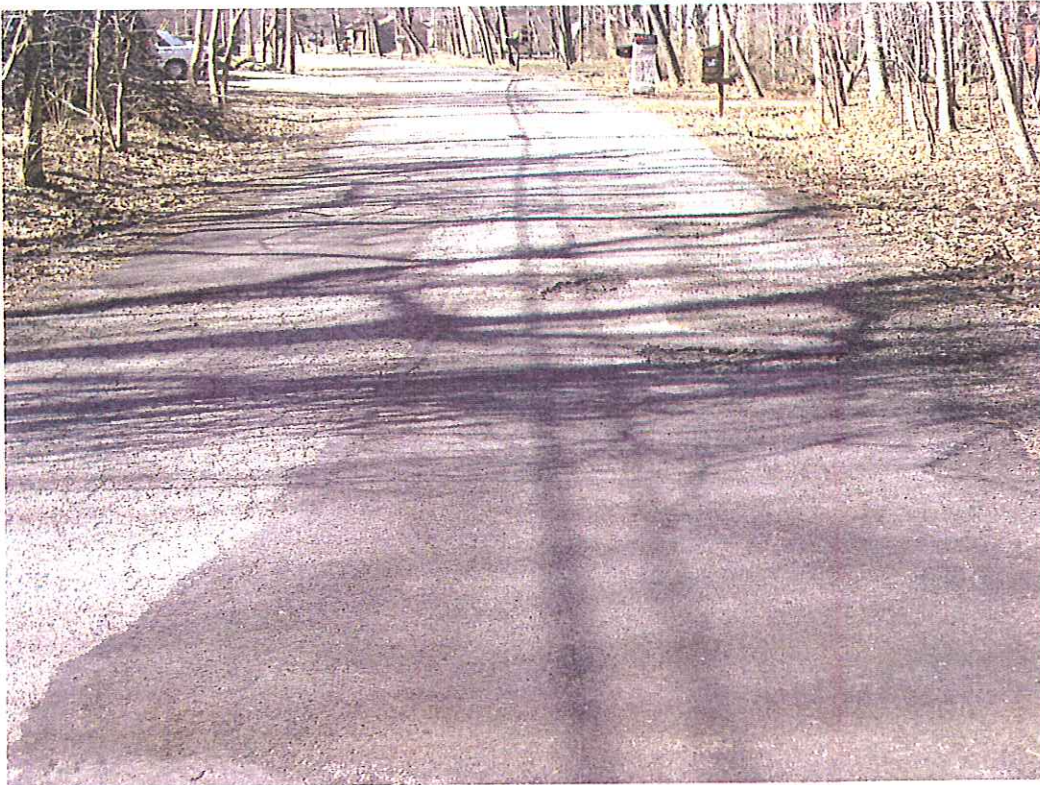
Picture 5 – Pavement Segment 311 (3168 Memorial Shoreway) CONDITION RATING NUMBER 1
