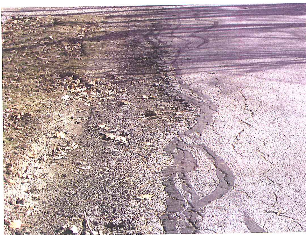
Picture 2 – Pavement Segment 405 (3021 South Confederate Drive)
