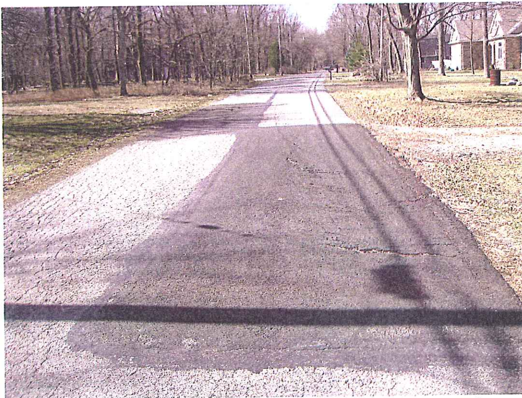
Picture 10 – Pavement Segment 317 (3274 Memorial Shoreway) CONDITION RATING NUMBER 1
