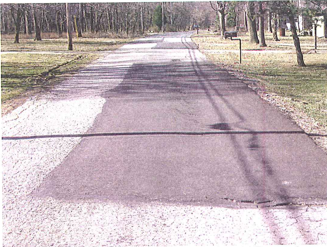
Picture 9 – Pavement Segment 316 (3254 Memorial Shoreway) CONDITION RATING NUMBER 1
