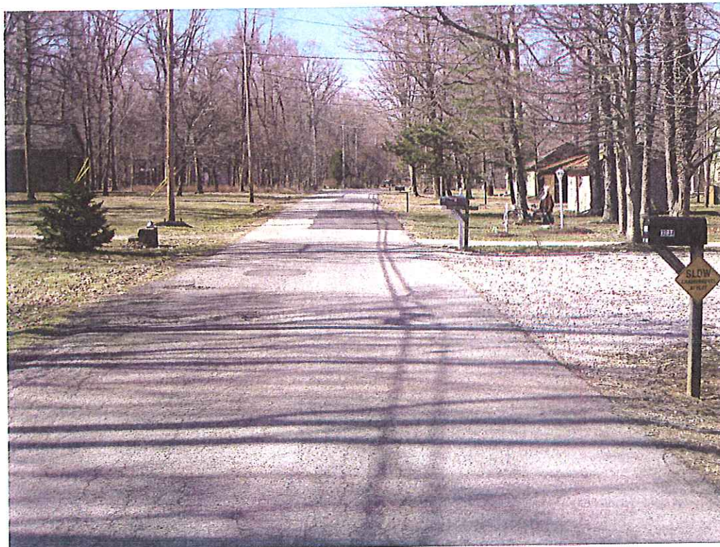
Picture 8 – Pavement Segment 311 (3234 Memorial Shoreway) CONDITION RATING NUMBER 1
