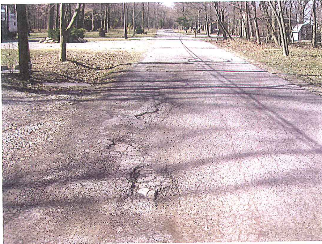
Picture 7 – Pavement Segment 313 (3206 Memorial Shoreway) CONDITION RATING NUMBER 1
