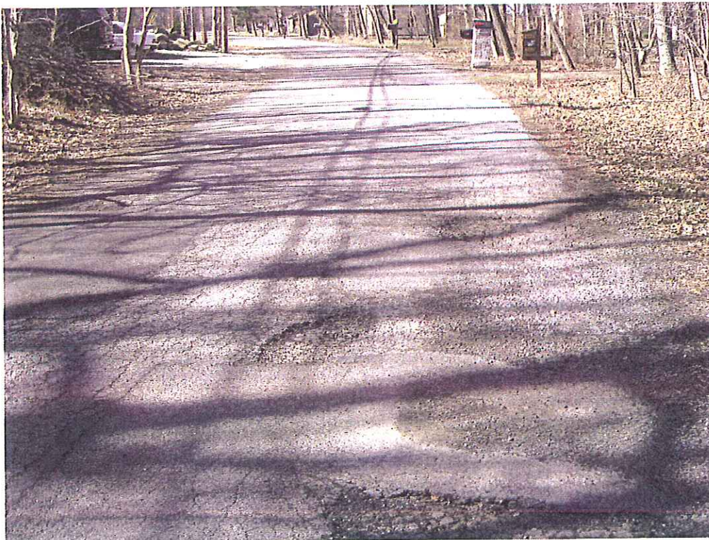
Picture 6 – Pavement Segment 311 (3182 Memorial Shoreway) CONDITION RATING NUMBER 1
