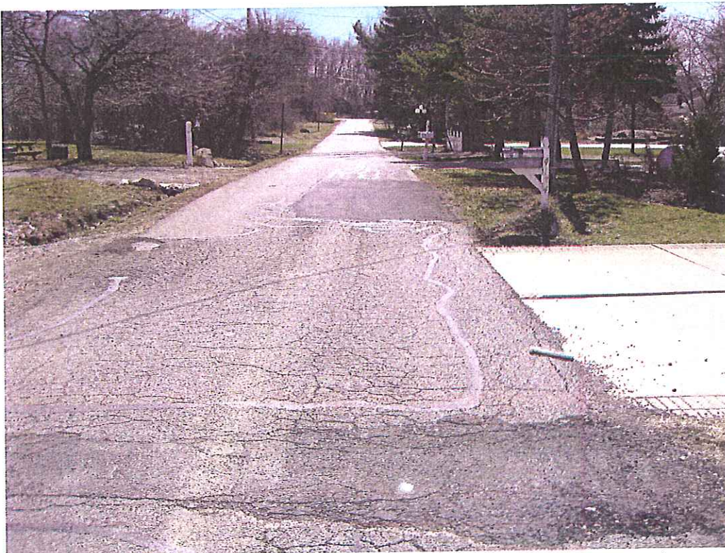
Picture 28 – Pavement Segment 356 (4134 Memorial Shoreway) CONDITION RATING NUMBER 6
