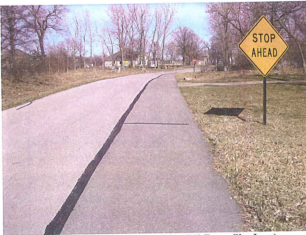
Picture 34 – Pavement Segment 701 (4370 Forest Glen Lane)
