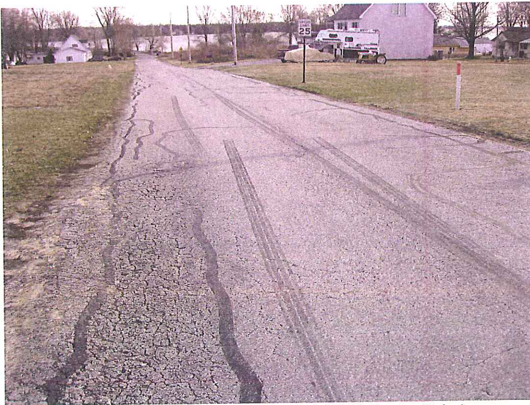
Picture 42 – Pavement Segment 101 (8076 Gaydos Drive) CONDITION RATING NUMBER 4
