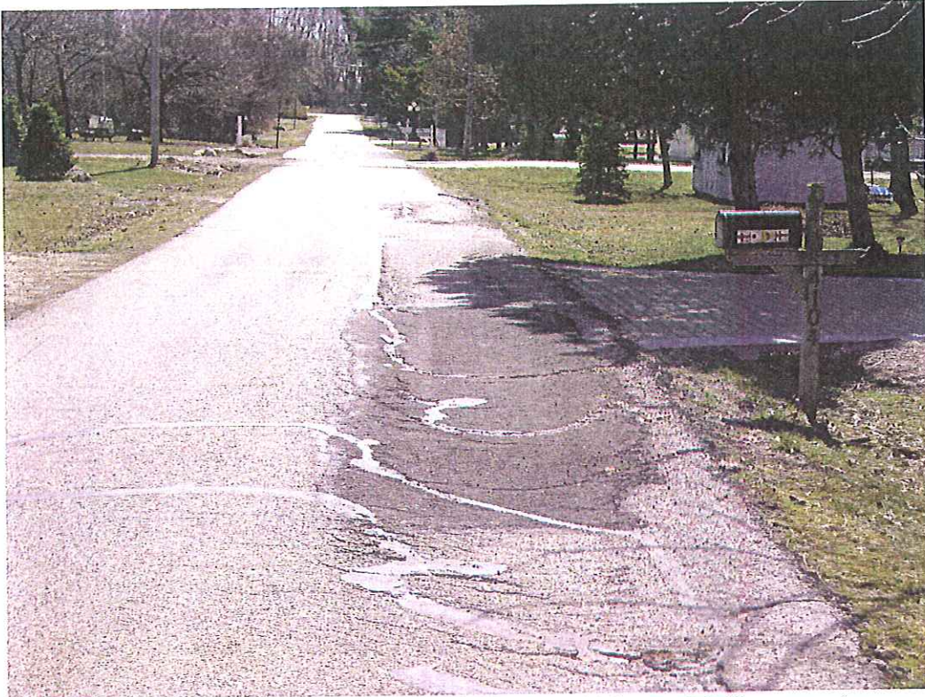
Picture 27 – Pavement Segment 355 (4094 Memorial Shoreway) CONDITION RATING NUMBER 6
