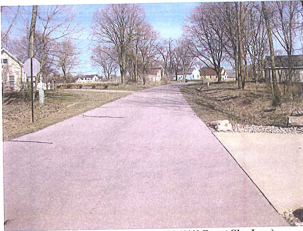
Picture 37 – Pavement Segment 703 (4460 Forest Glen Lane)
