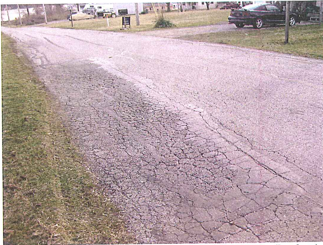
Picture 41 – Pavement Segment 101 (Gaydos Drive south from Bayshore) CONDITION RATING NUMBER 4
