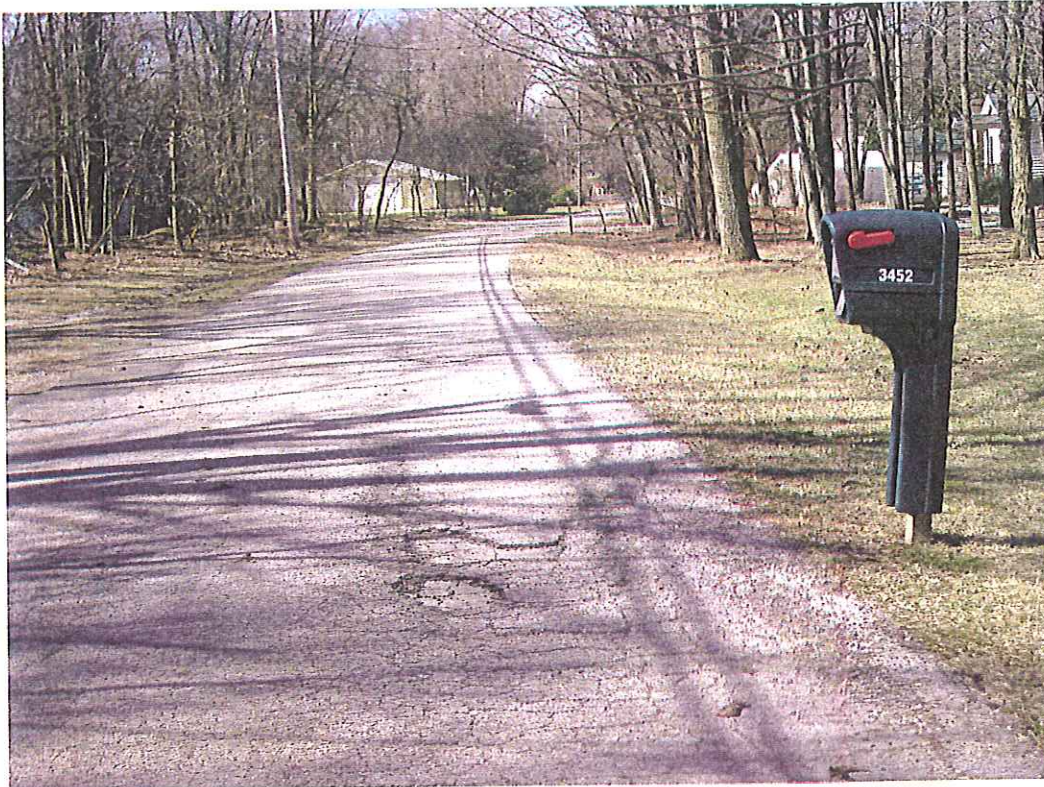
Picture 15 – Pavement Segment 326 (3452 Memorial Shoreway) CONDITION RATING NUMBER 5
