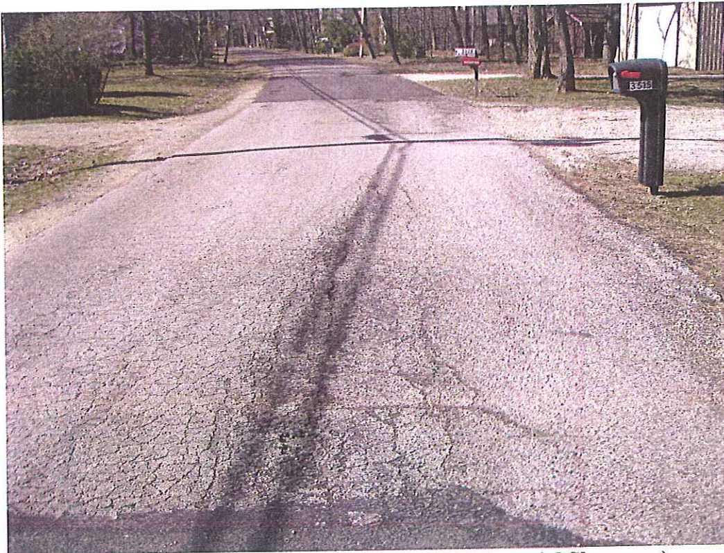
Picture 18 – Pavement Segment 329 (3510 Memorial Shoreway) CONDITION RATING NUMBER 5
