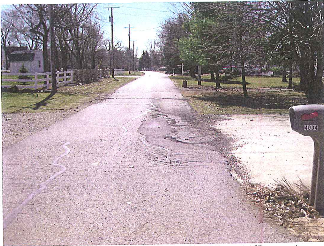
Picture 25 – Pavement Segment 349 (4004 Memorial Shoreway) CONDITION RATING NUMBER 7
