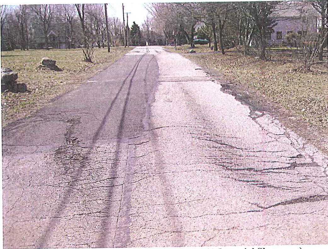
Picture 21 – Pavement Segment 337 (3694 Memorial Shoreway) CONDITION RATING NUMBER 2
