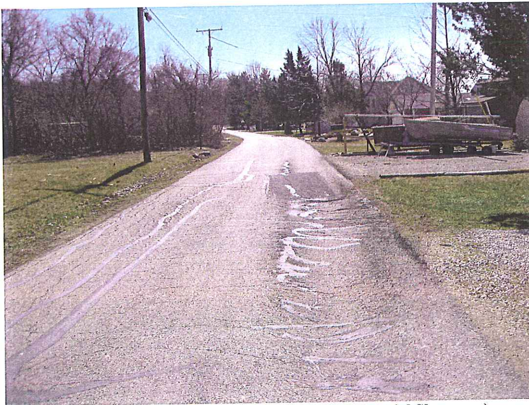
Picture 26 – Pavement Segment 353 (4064 Memorial Shoreway) CONDITION RATING NUMBER 6
