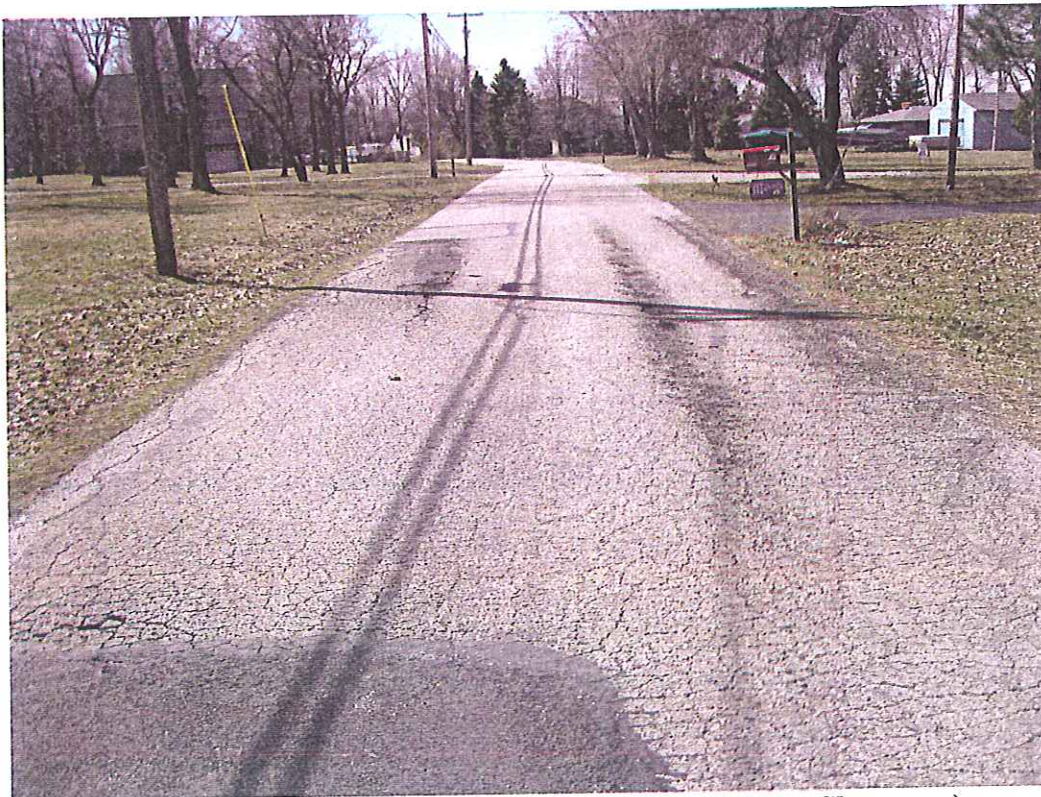
Picture 22 – Pavement Segment 338 (3734 Memorial Shoreway) CONDITION RATING NUMBER 2
