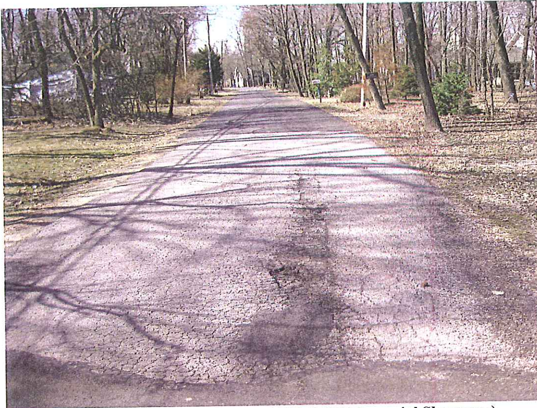
Picture 19 – Pavement Segment 331 (3528 Memorial Shoreway) CONDITION RATING NUMBER 5
