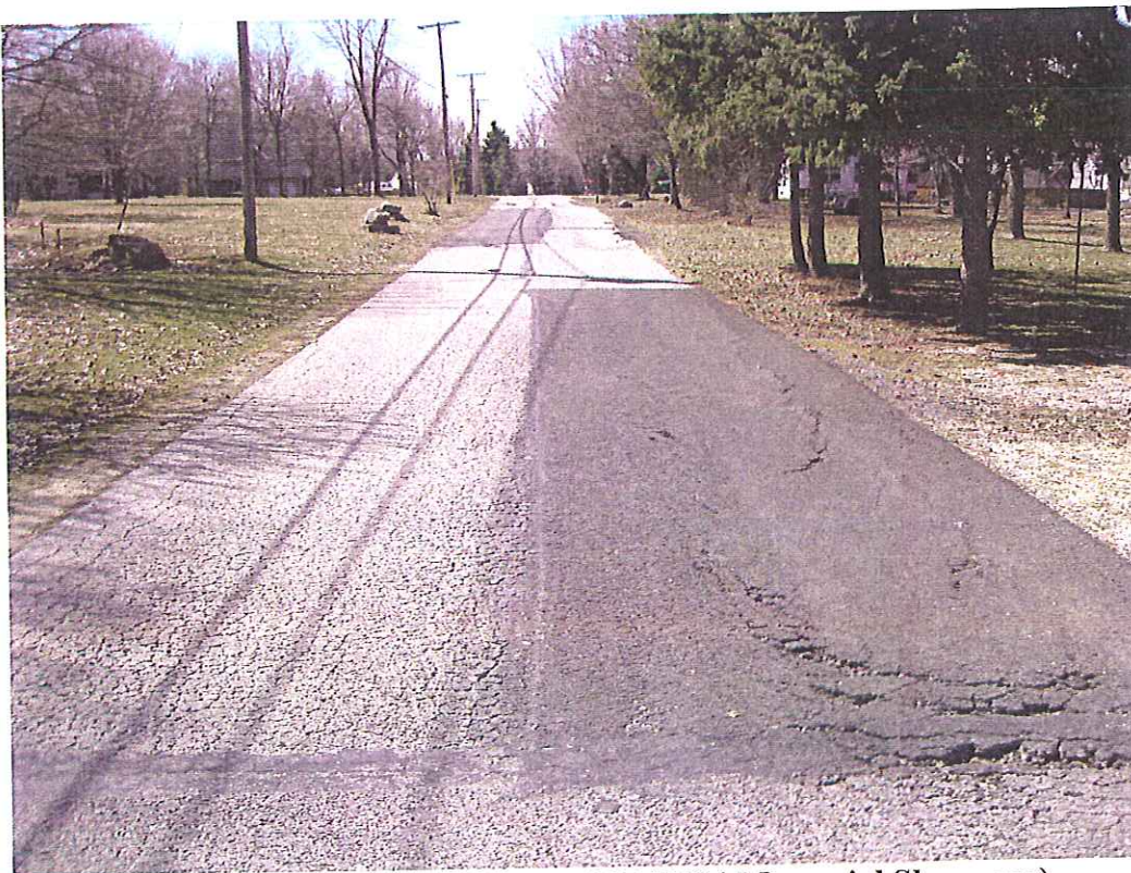
Picture 20 – Pavement Segment 337 (3694 Memorial Shoreway) CONDITION RATING NUMBER 2
