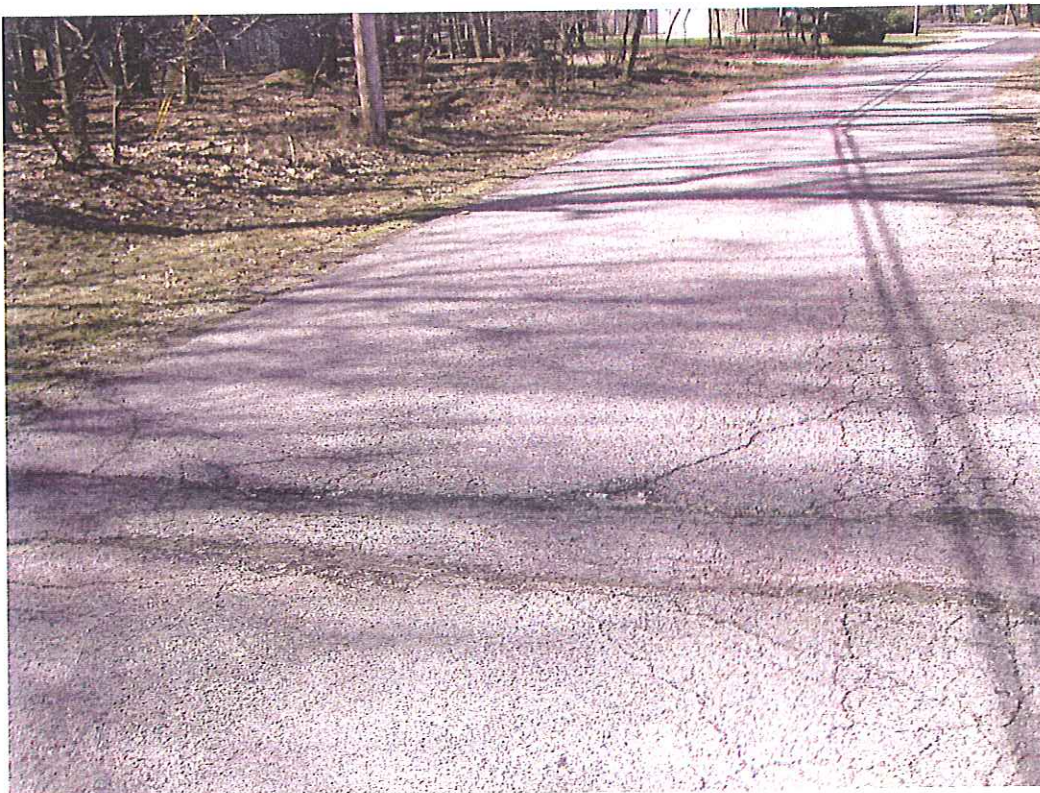
Picture 16 – Pavement Segment 326 (3452 Memorial Shoreway) CONDITION RATING NUMBER 5
