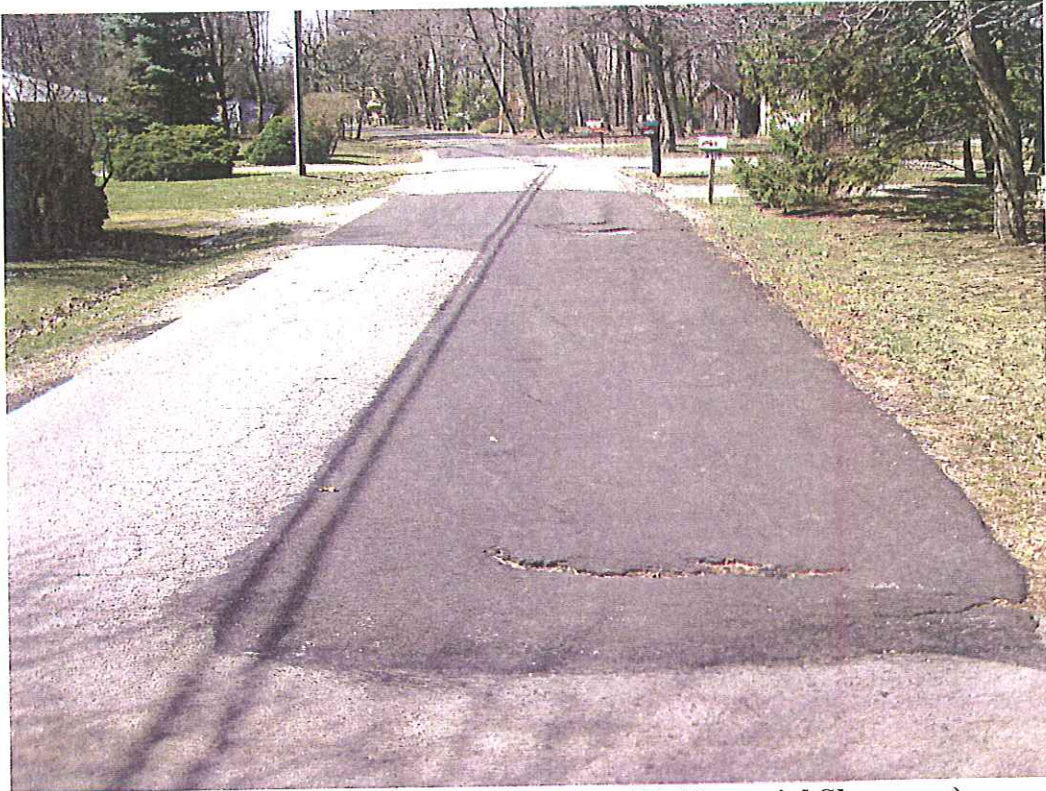
Picture 17 – Pavement Segment 328 (3492 Memorial Shoreway) CONDITION RATING NUMBER 5
